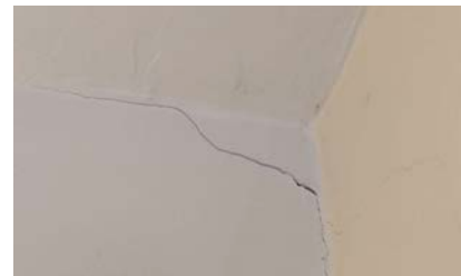
Figure 4. Crack in my LA apartment (Van Auken, 2019).
