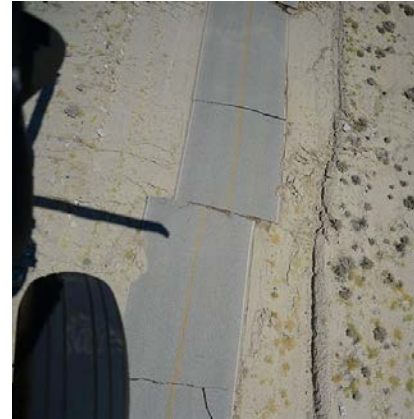
Figure 3. Road damage resulting from 3 to 5 feet of right-lateral motion (USGS, 2019).
